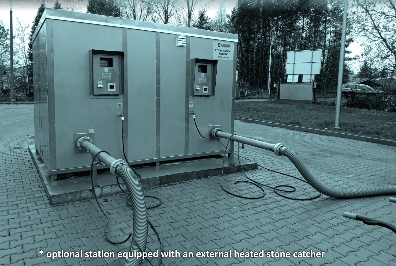
Wastewater disposal station STZ
