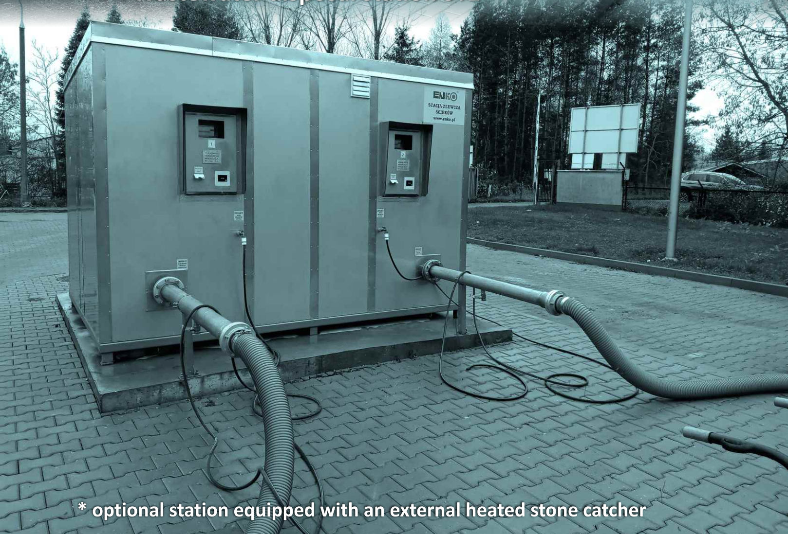
Wastewater disposal station STZ
